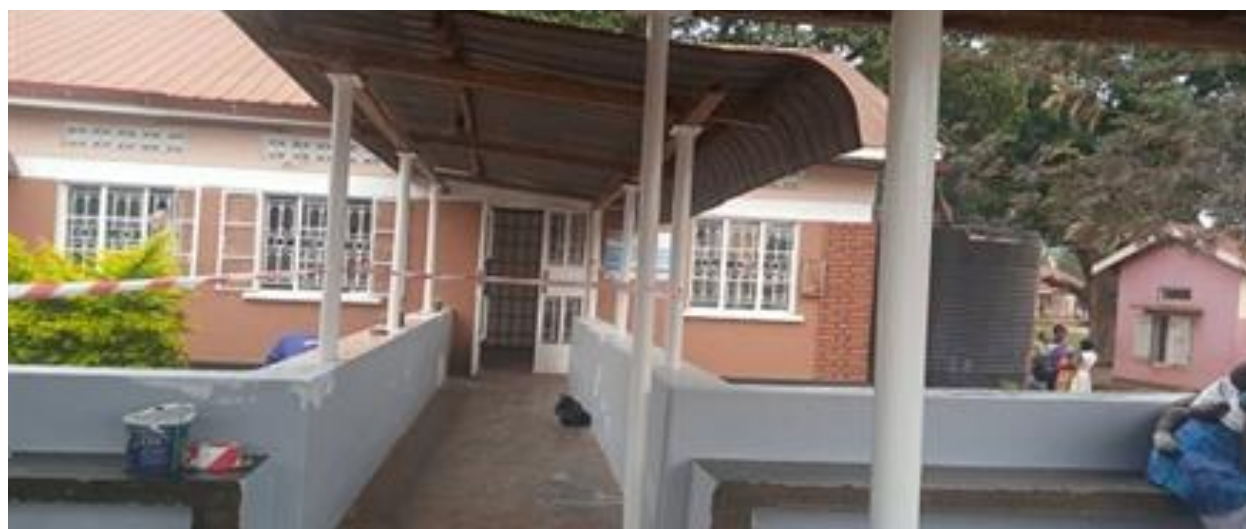
Renovation of OPD block at Kasangati HC IV by Opportunity Buddy group Kyanjja
